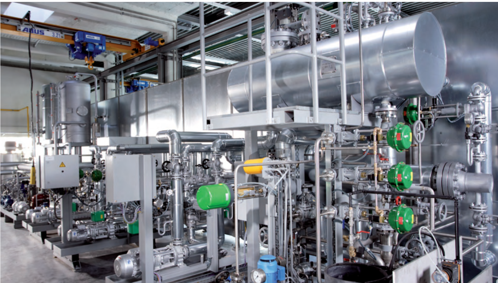
R&D laboratory – heating center for media
